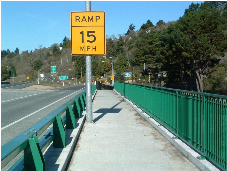
Type ST-10 (left) and Metal Pedestrian Railing (right) at Mad River Bridge
