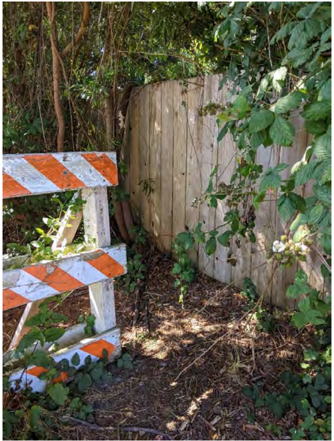
Photos 9-10. West Bates Road and Thiel Ave. Barrier should be modified to allow bike-ped access.
