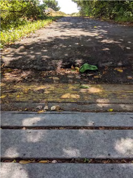
Photo 2. Strawberry Creek Bridge South Footing. Wood or rubber ramp needed.
