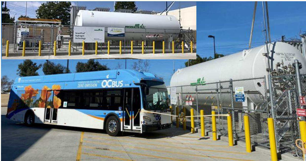
Figure 6: Picture of Orange County Transit Authority's 4,500 kg liquid hydrogen storage and fueling infrastructure constructed in 2020. Station footprint inside the bollards is roughly 40' x 80'. This does not include required code setbacks or fuel dispensers and required chillers. This equipment is located on a separate fueling station island and is roughly the size of a typical diesel fuel pump. Images from trilliumcng.com and tass.news .
