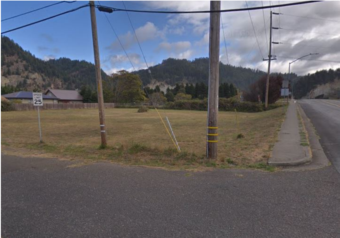
Figure 6: Sidewalk Terminates at the intersection of Davis St. and Ireland St. (No crosswalk or ADA ramps)
